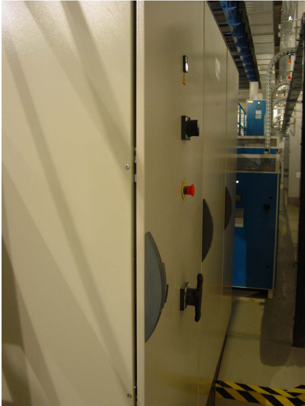
ARMOIRE GENERALE TRAITEMENT DE SURFACE
